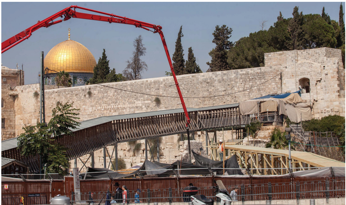
Demolitions of historic remains and continued excavations at the Magharbeh Gate Pathway.
