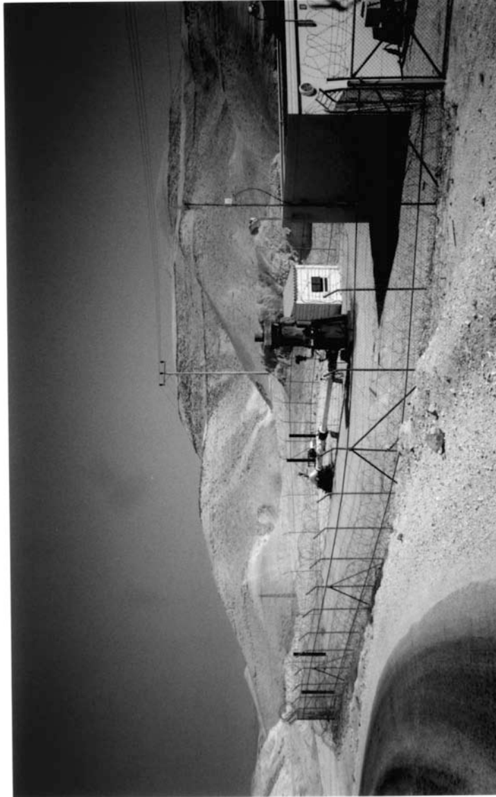
One of many Israeli water pumping stations in the West Bank used to extract water for Israeli consumption (including settlements). Some 82% of West Bank water is used in this manner.
